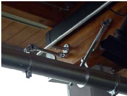
Lateral and Longitudinal Sway Braces
